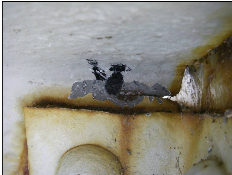
Figure 10b – Fatigue crack in floorbeam web above clip angle to inboard lower chord truss. 1-5/8" long on 8/6/09
