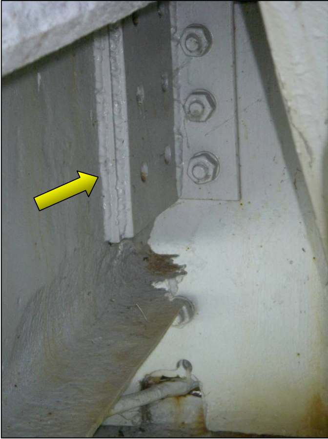
Figure 7 - Vertical weld on right fascia stringer web retrofit at end Floor beams (0 and 9)
