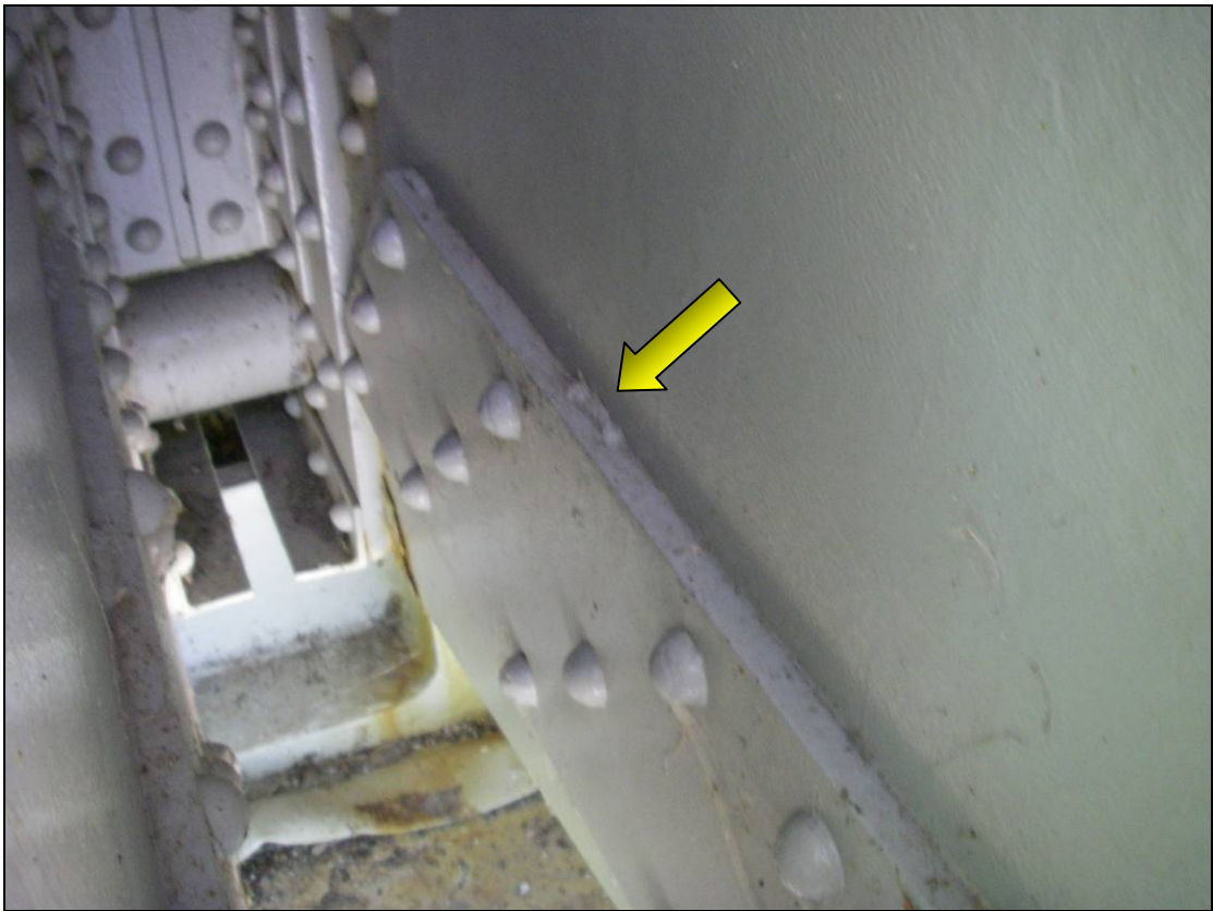
Figure 4a - Tack weld connection at Gusset Plate to Lower Chord flange plates
