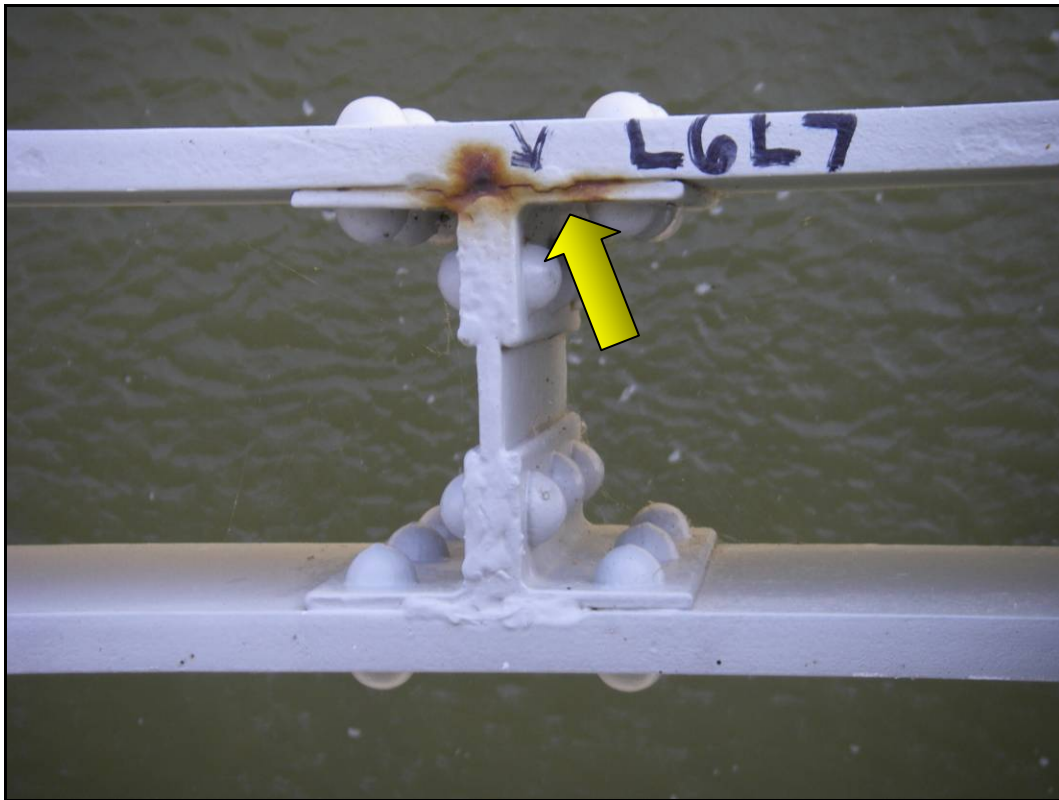
Figure 8b - Tack welds on web-plate diaphragms between lower chord flange plates. Location: Right truss span 4, L6L7, note crack around angle-fusion zone of tack weld
