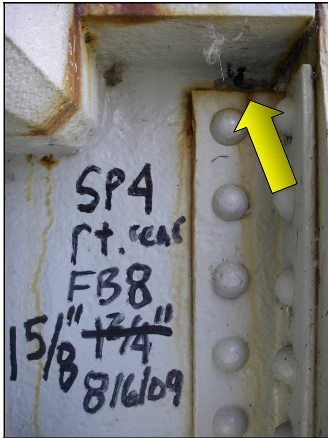
Figure 10a – Fatigue crack in floorbeam web above clip angle to inboard lower chord truss. 1-5/8" long on 8/6/09
