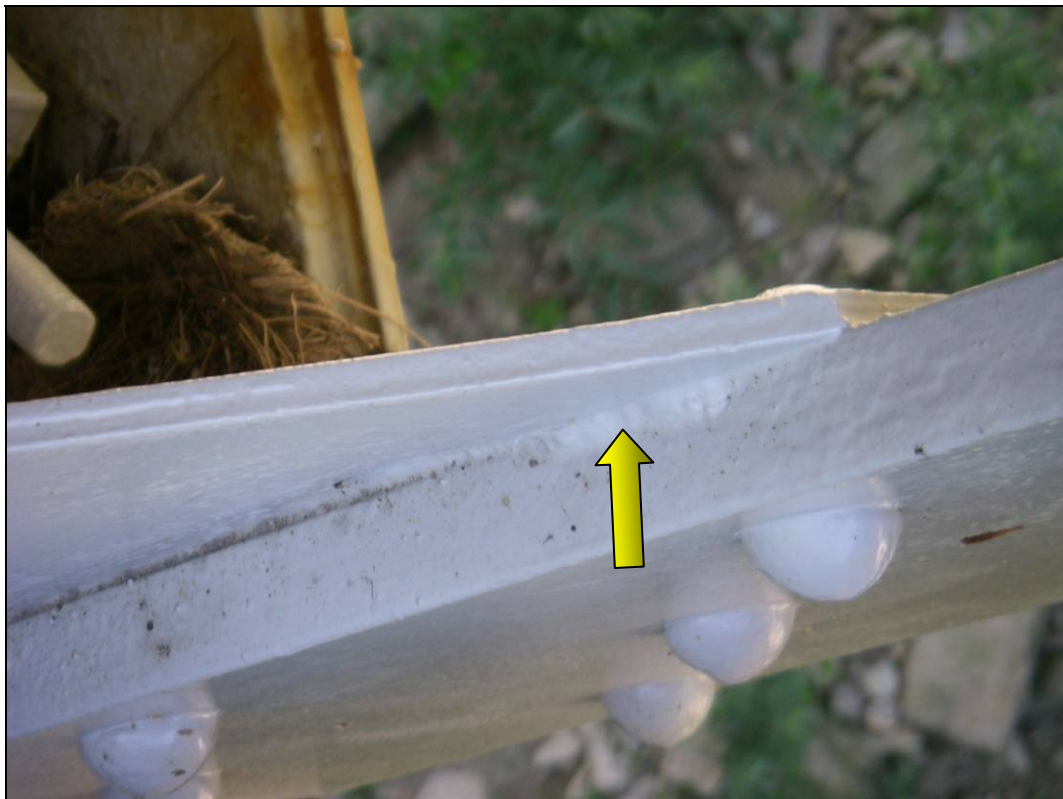
Figure 4b - Tack weld connection at Gusset Plate to Lower Chord flange plates
